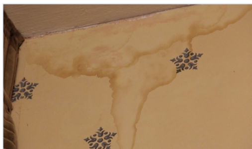
Building water damages
